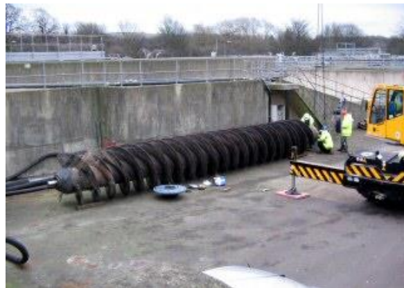
Figure 1-10: Screw removed for maintenance at a WWT plant
